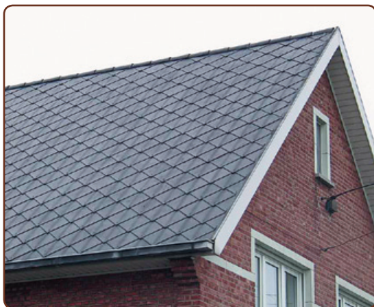
Dakleien in asbestcement
